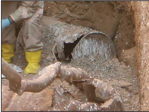
Figure 20. Sloping trenches with exposed drums and debris.
