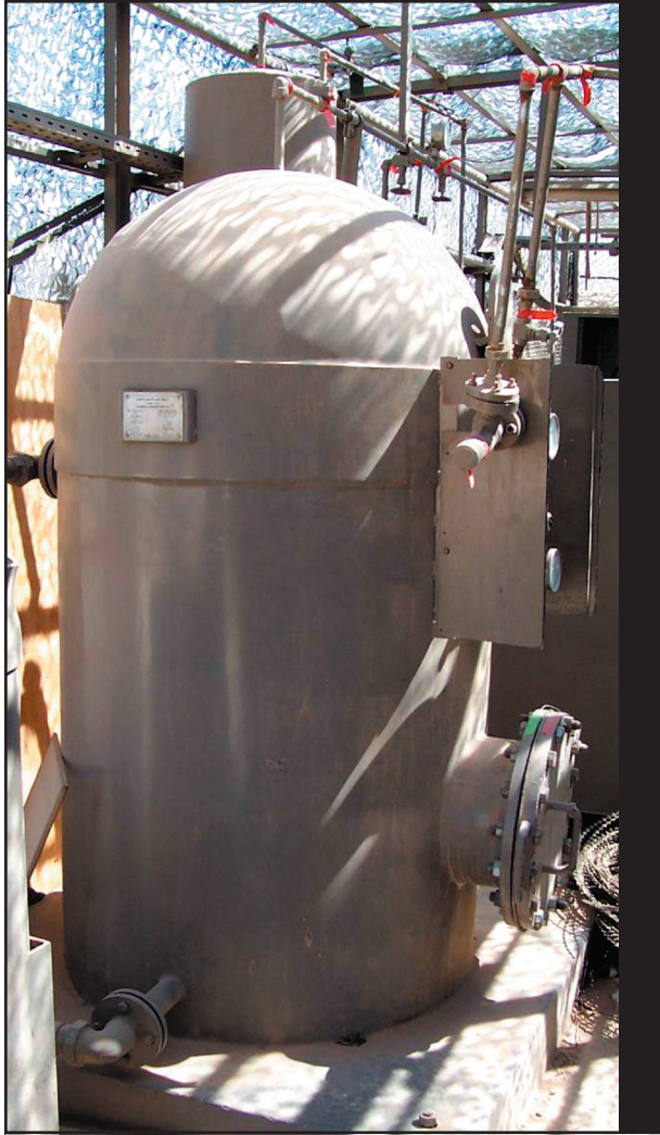
Figure 3 (a). Trailer 1 reactor vessel.
